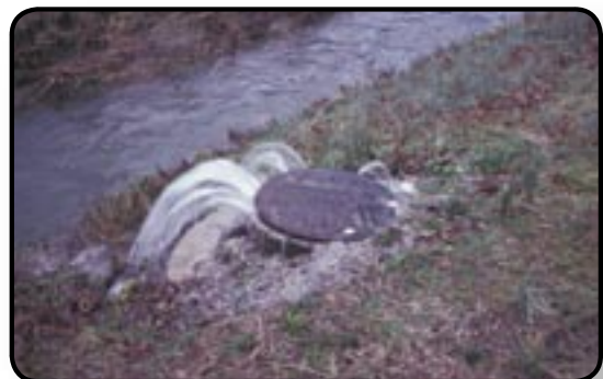
Stormwater infiltration causes sanitary sewer to overflow.
